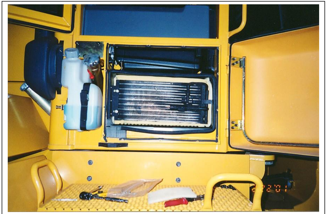
Evaporator assembly in place.
